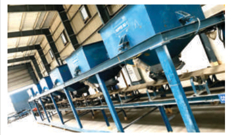
AUTOMATIC RAW MATERIAL BATCHING SYSTEM
